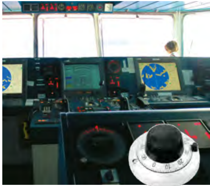
Panels on rig control house
